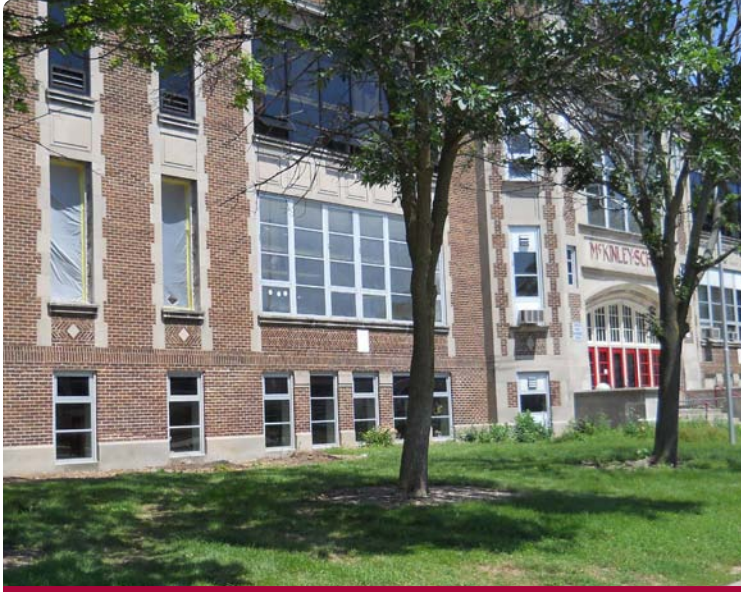
BEFORE: 1950s-era windows in the process of being replaced at McKinley Middle School
