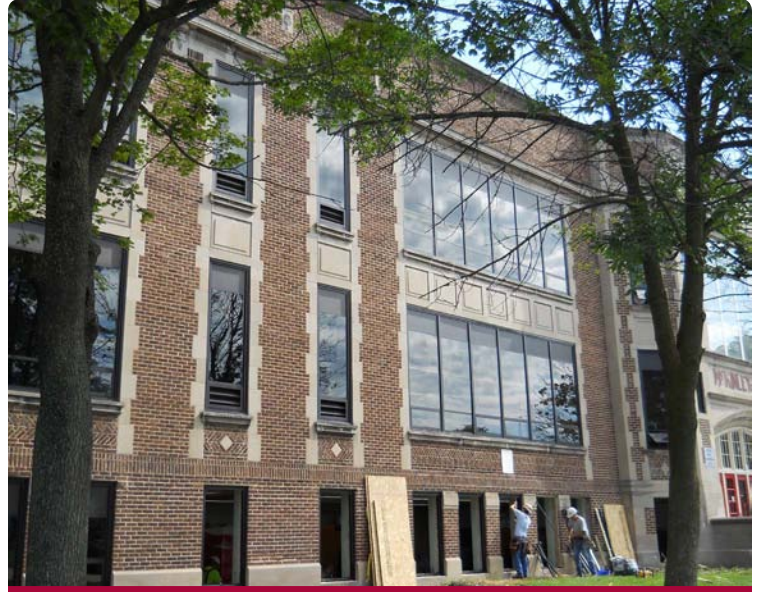
AFTER: Windows at McKinley Middle School are replaced with new energy-efficient windows.
